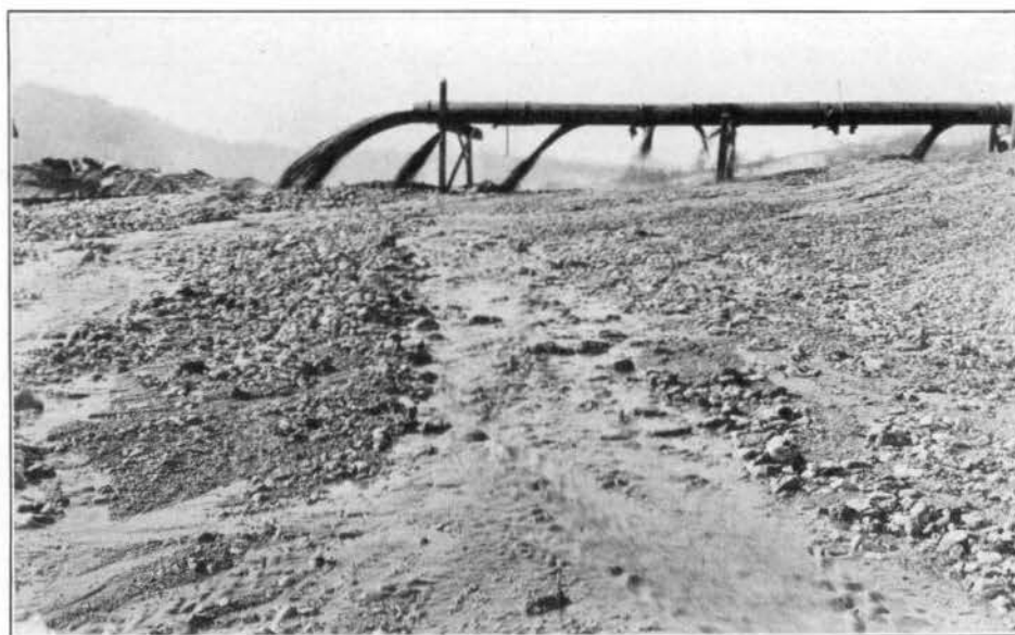
FIG. 94—GERMANTOWN WINDOW PIPE, ANOTHER VITW, JAN. 28, 1920
