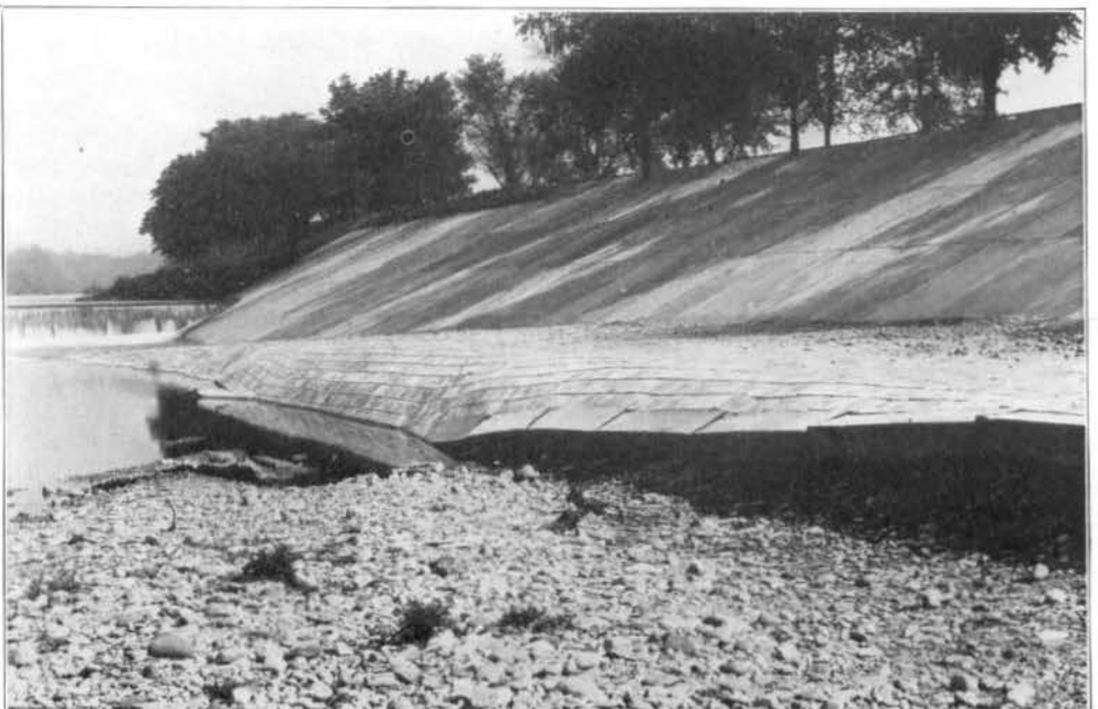
FIG. 145—FLEXIBLE REVETMENT AFTER APRIL FLOOD. MAY 26, 1920.
