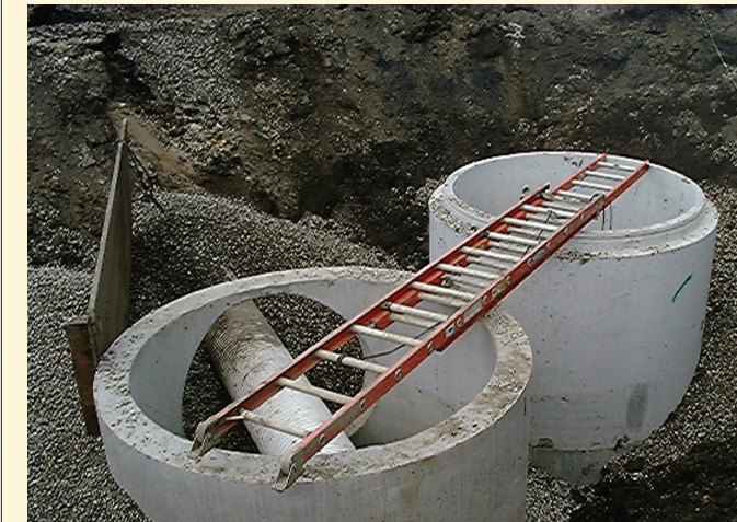
The primary manhole is installed in-line with the storm drain (left unit) alongside the storage manhole (right unit).
