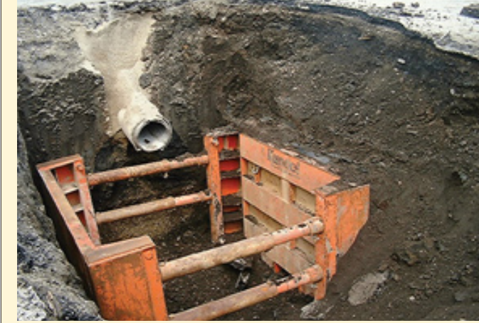
Construction of the Separator System shows the excavation site at the parking facility.
