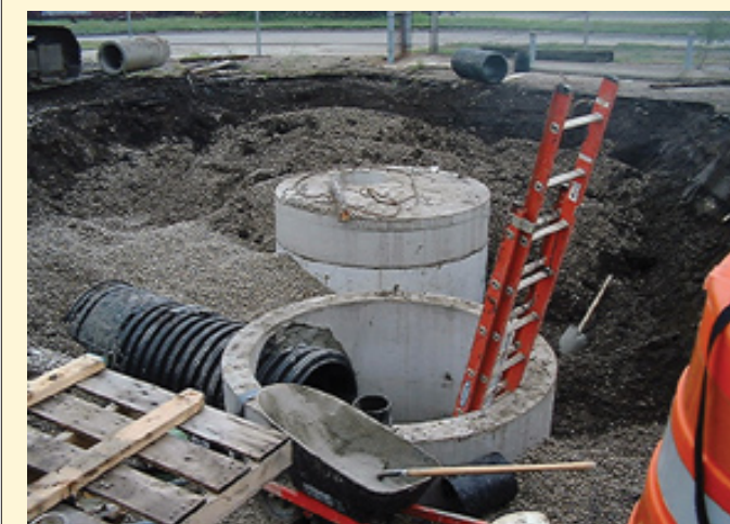
Both manholes are capped, and backfill aggregate is installed around each unit.
