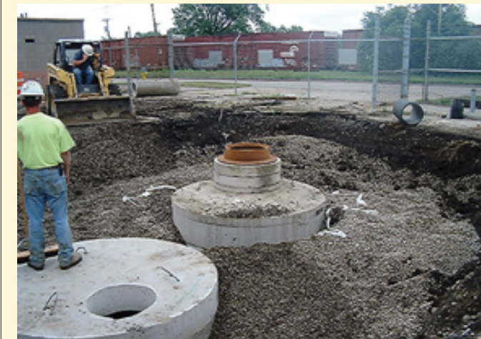
The BaySaver Separator System shows final backfill, with grading and surfacing to be completed.
