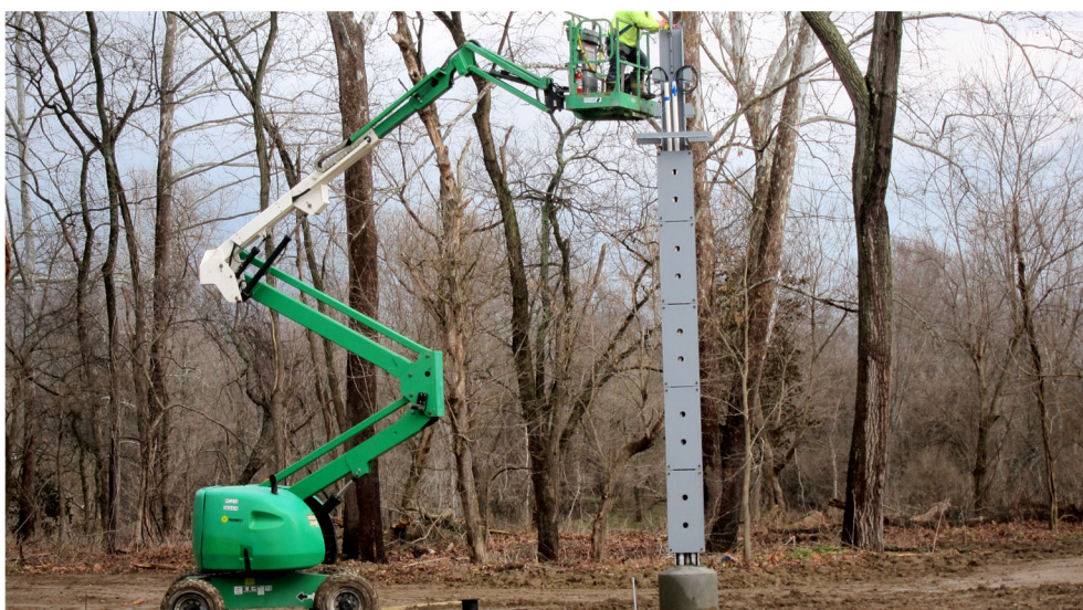
Installing a pylon to store and transmit groundwater data collected at THEMMS.
